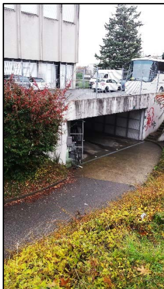
Figure 3: Beneath the Department of Public Instruction of Culture and Sport in Geneva
